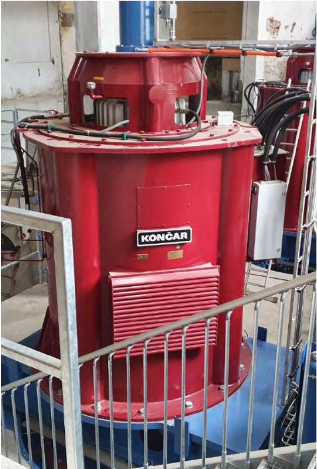
New compact generator for HPP Haunoldmühle in Austria
