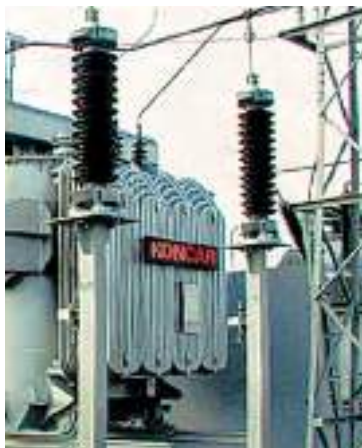
Single-phase power transformer
