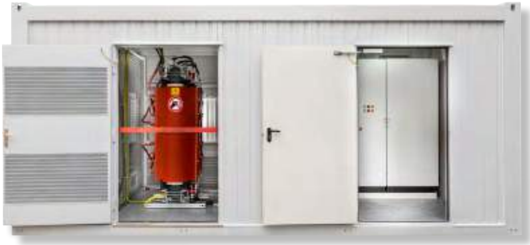
KonSol – converter equipment in a container at a PVPP project in Croatia
